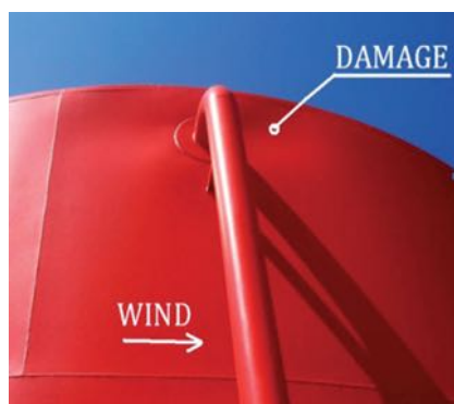
Figure 9 - Damaged Water Tank Riser
