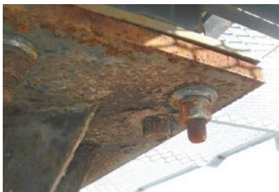
Figure 16 - Structural Condition of Billboard Connections
