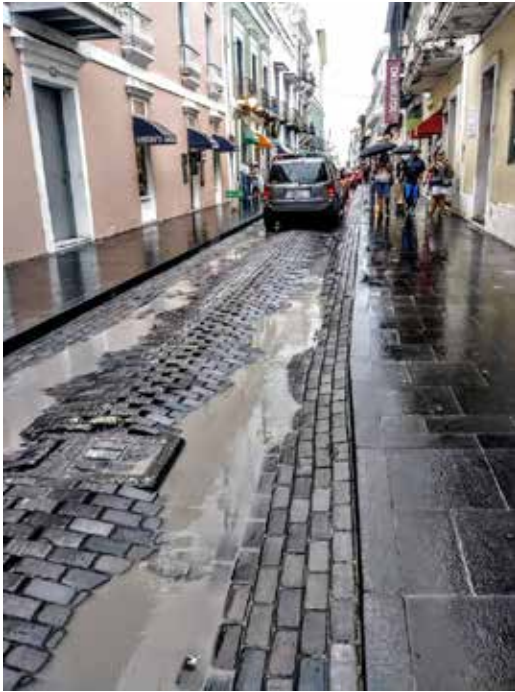
Figure 7. La Fortaleza street collapsing after questionable reconstruction processes enabled by the Municipal Government of San Juan. (Photo: Andrés Rivera, PRHBS, 2016)
