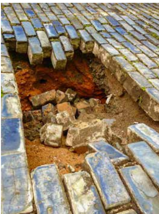
Figure 3. The continued traffic over the historic streets in El Viejo San Juan is causing the collapse of the bricked streets and its underground tunnel systems developed in the second half of the 19th century. (Credits: Andrés Rivera, PRHBS, 2019)
