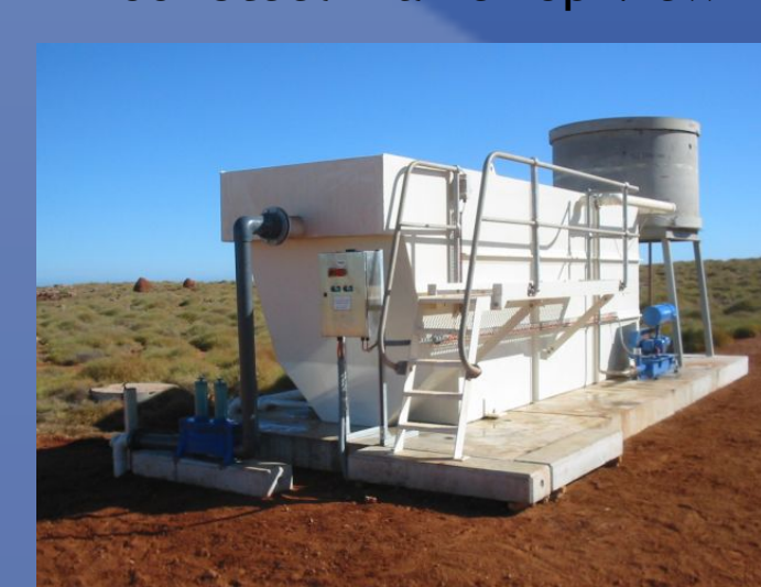
Wastewater Package Treatment Plant
