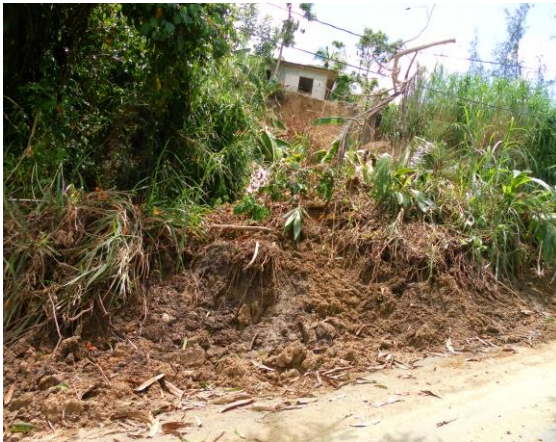
Figure 3 Landslide Movement (Front View)
