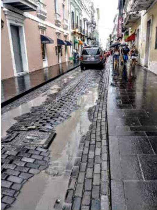
Figure 7. La Fortaleza street collapsing after questionable reconstruction processes enabled by the Municipal Government of San Juan. (Photo: Andrés Rivera, PRHBS, 2016)
