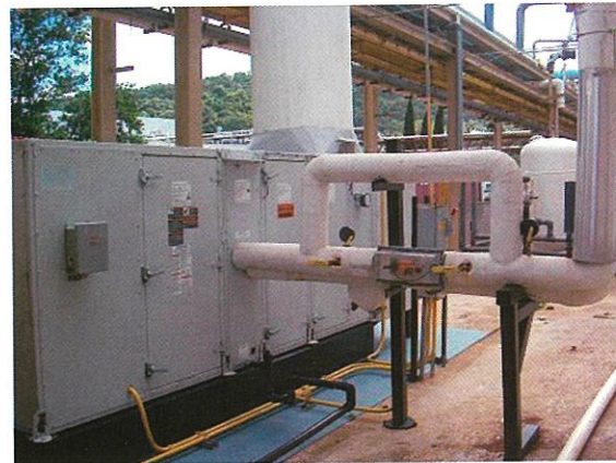
Figure 1: AHU Considered for Economizer Implementation
