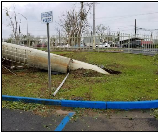
Figure 4 Yielding or Inelastic Buckling Failure, Bayamon P.R.
