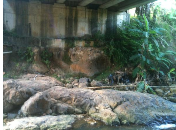
Figure 8 Scour at Right Abutment
