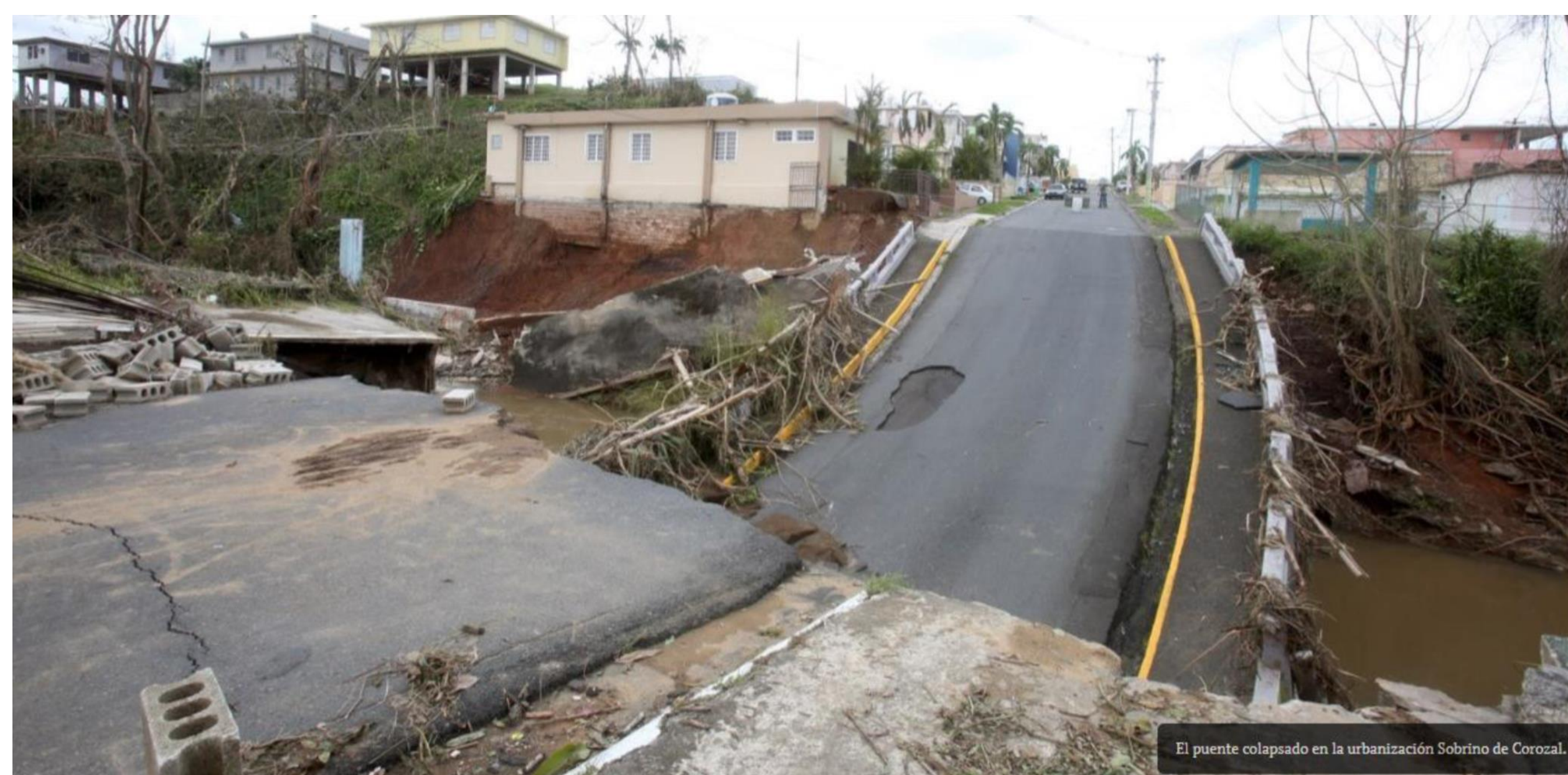
Figure 1: Fallen Bridge in Corozal, Puerto Rico (Cruzado & Pacheco, 2018)
