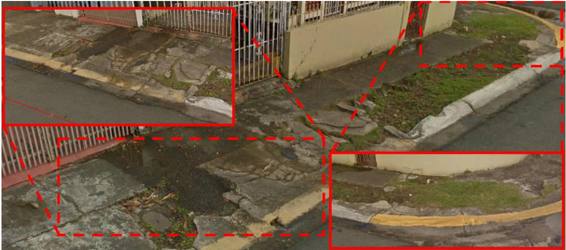
Figure 6-211 Damage of Sidewalk on East Street from the Evacuation Route of Francisco Oller (Google Earth – 2016)
