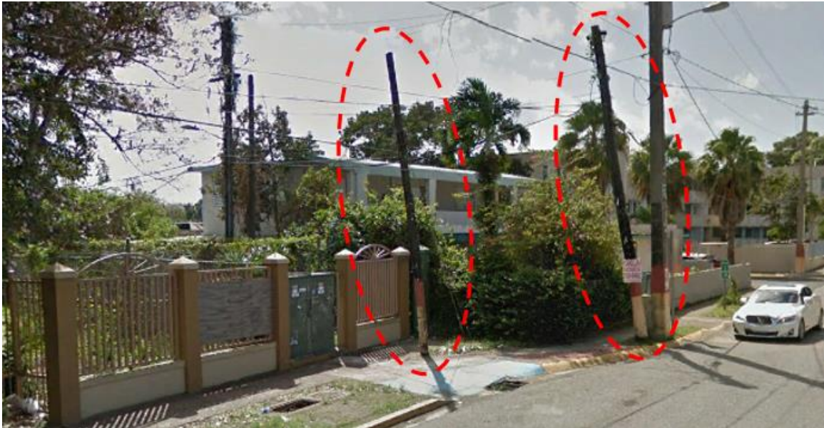
Figure 6-216 Poles with Power Lines in First Section of Sidewalk on Las Nereidas Avenue from the Evacuation Route of Francisco Oller School in Street View (Google Earth - 2016)
