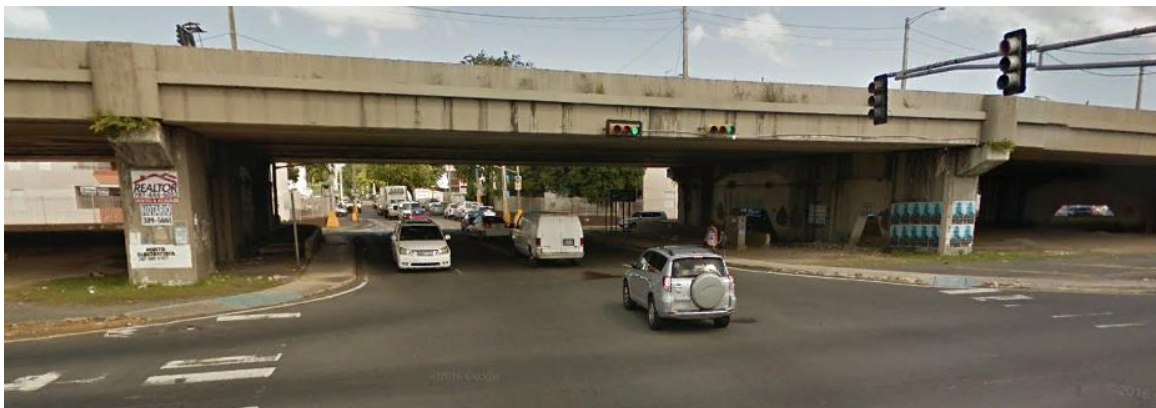
Figure 6-284 Bridge on the Evacuation Route of Luis Llorens Torres School (Google Earth – 2016)
