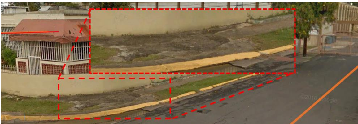
Figure 6-207 Damage of Sidewalk on Central Street from the Evacuation Route of Francisco Oller (Google Earth – 2016)
