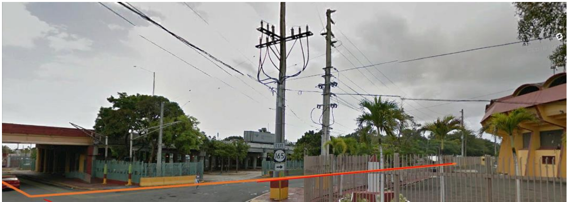
Figure 6-202 Power Lines on the Evacuation Route of Francisco Oller through José Celso Barbosa Avenue School (Google Earth – 2016)
