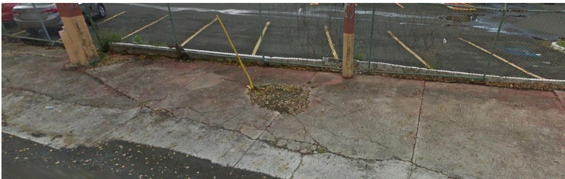
Figure 6-230 Sidewalk Damage on Olivo Street from the Evacuation Route of Francisco Oller School in Street View (Google Earth – 2016)
