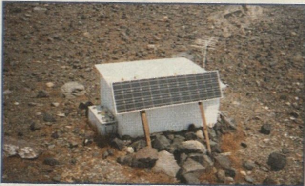
Seismometer (in the white box), solar panel & telemetry for monitoring volcanic activity in near-real time.
