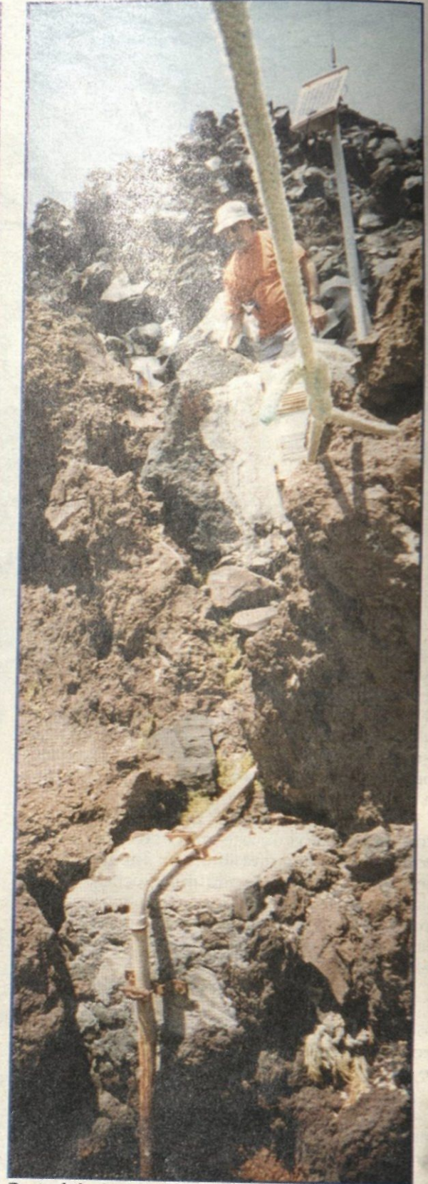
Part of the installed tide gauge (instrument to monitor the variations on the sea level), solar panel & telemetry.
