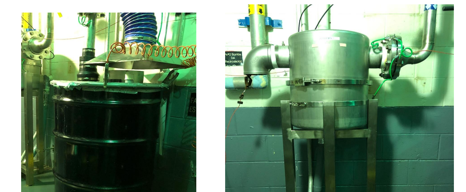
Figure 7: Suspended Hood and HEPA Filter Station
