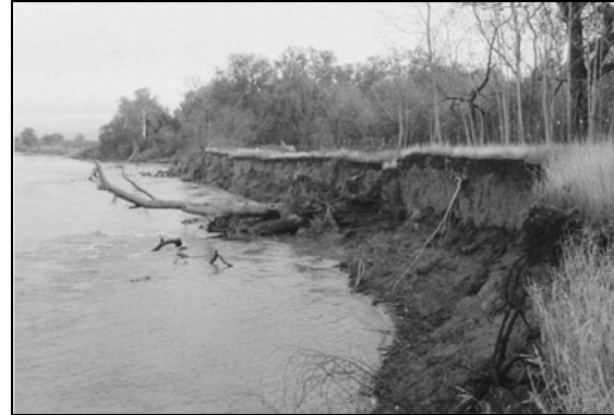
Figure 3 Active Bank Erosion Illustrated by Vertical Cut Banks
