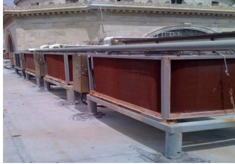
Picture 2 Existing A/C units at the roof.
