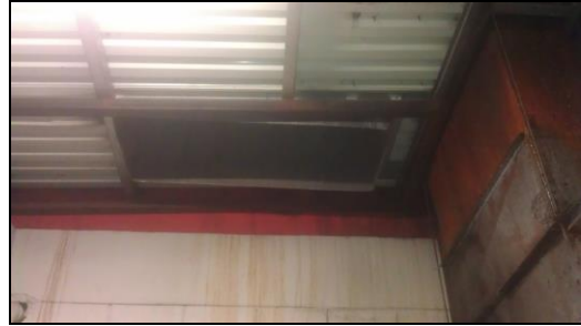
Figure 3 Actual common return air
