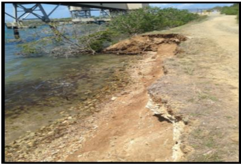
Figure 3 Harbor road erosion
