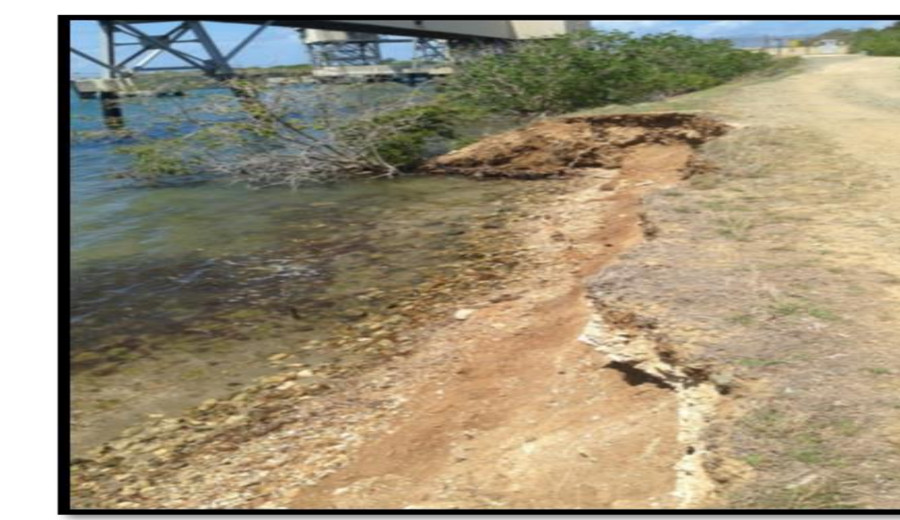
Figure 3 Harbor road erosion
