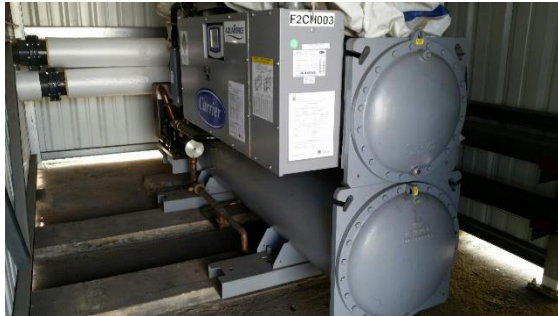
Figure 9 Water-Cooled Chiller Installed
