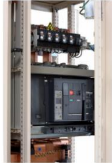
Figure 2 Fixed breaker (inside a cradle) in Switchboard gear.
