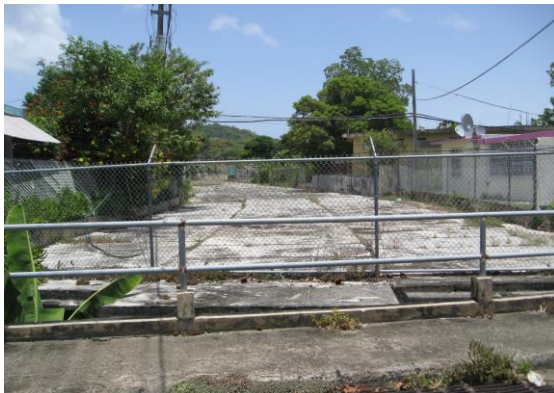
Figure 6 Box Culvert at Quebrada Mabu that has to be eliminated
