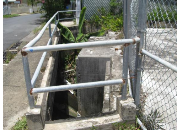
Figure 7 Box Culvert at Quebrada Mabu that has to be eliminated
