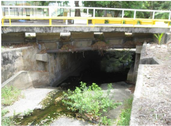
Figure 5 Bridge that has to be replaced on Quebrada Mabu
