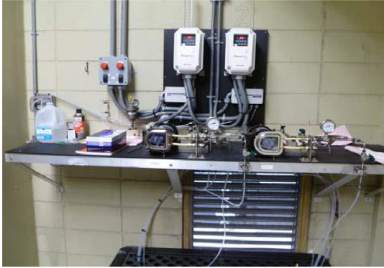
Figure 6 Peracetic Acid Pumps Skid
