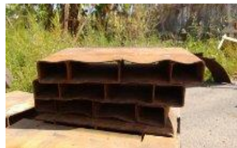
Figure 8 Boiler's Burner Components (3 years of use)
