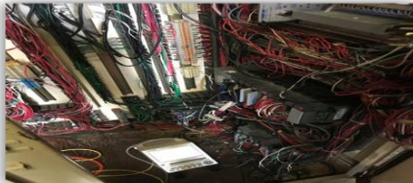
Figure 1 Pictures Showing Examples of the current Control System
