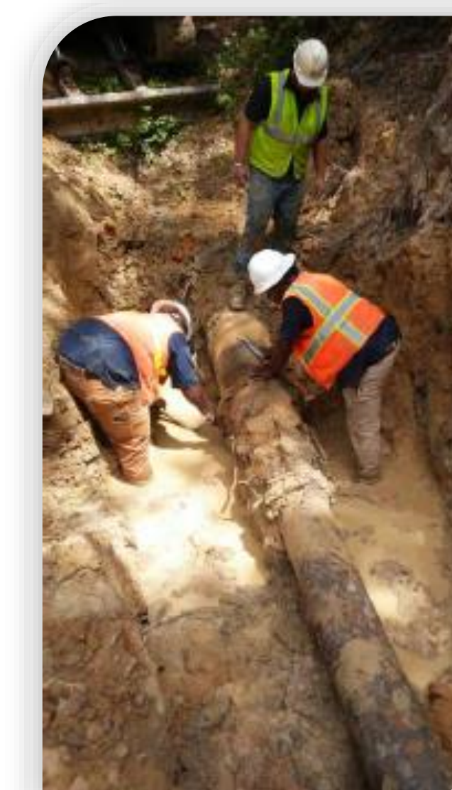
Figure 3 Marietta St Water Main Break Government Owned
