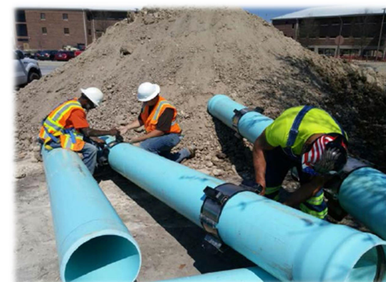
Figure 2 Sumter Ave. Water Main Break Private Contractor Owned
