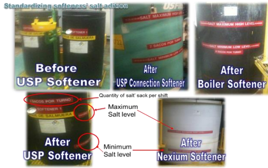
Figure 7 Visual Aids – Softeners Tanks
