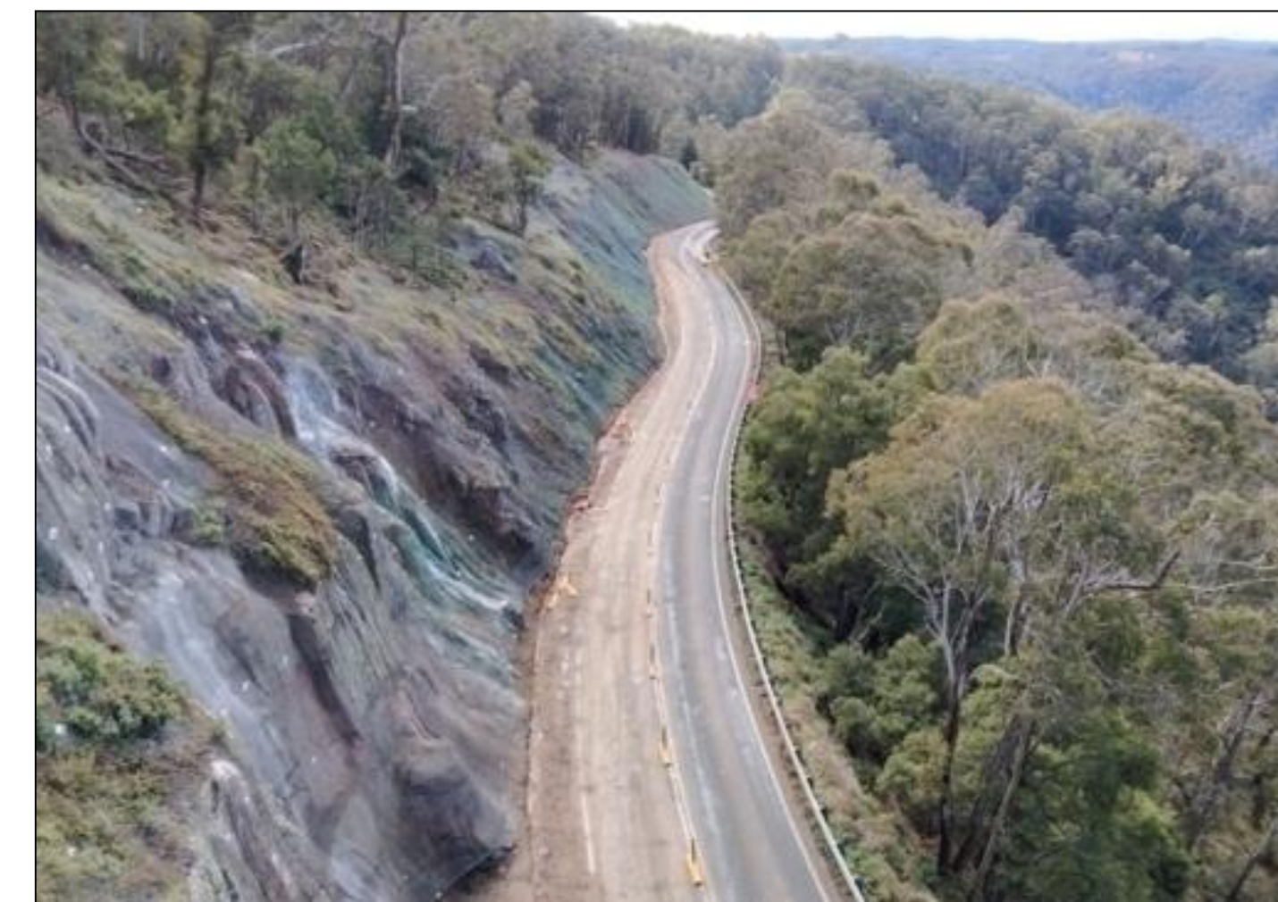
Wire Mesh Facing Over Rock Slope Example
