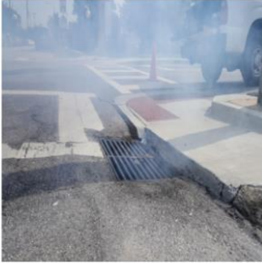
Figure 6 Combined System Identified During Smoke Test [7]
