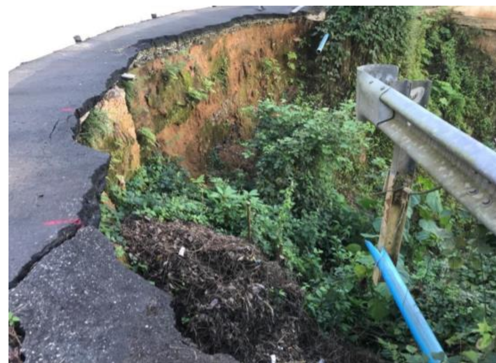
Figure 2. Shows the Slope Failure on PR-124
