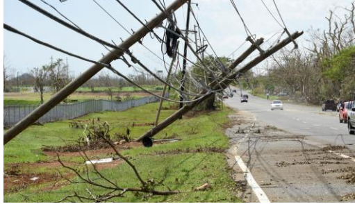
Figure 7 Damaged Poles in Barceloneta
