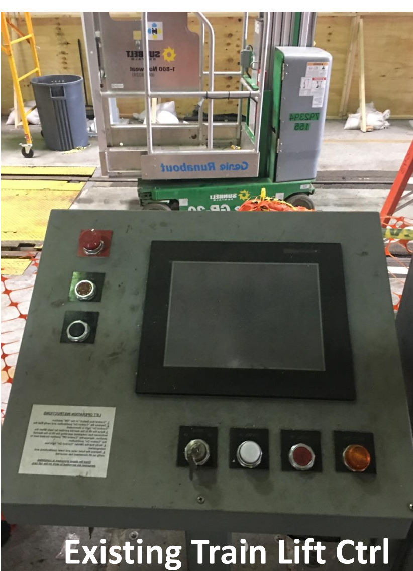
Existing Train Lift Ctrl
