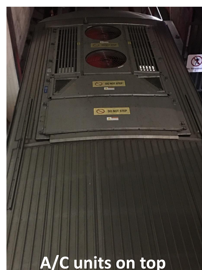
A/C units on top
