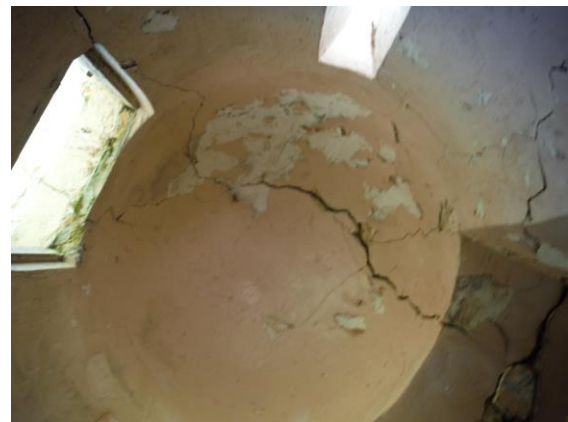
Figure 7 Substantial Crack inside the Half Dome of the Sentry Box
