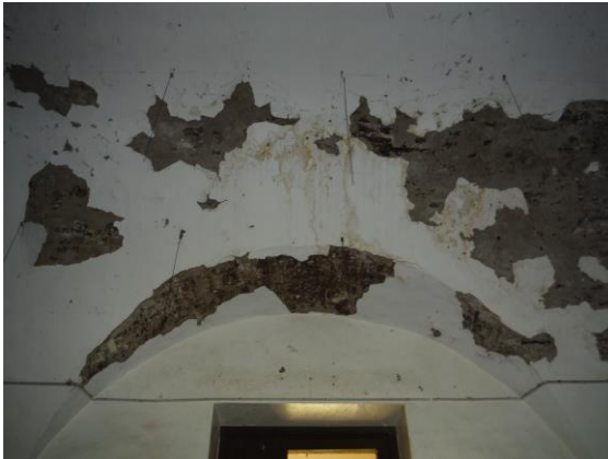
Figure 5 Barrel Vault Missing Concrete Cover
