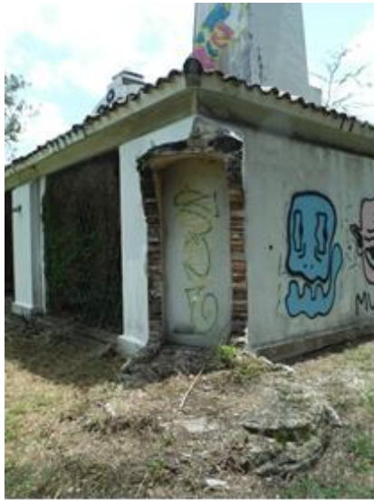
Figure 8 Missing Sentry Box
