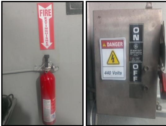
Figure 9 Safety – Fire Extinguisher & Voltage Label
