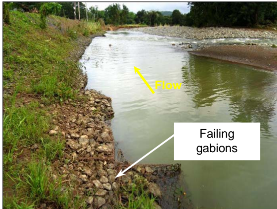
Figure 8 Failing Gabions on Río Mameyes, PR (2004)
