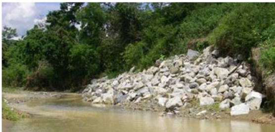
Figure 9 Riprap used for Streambank Erosion (Río Caguaitas, PR)
